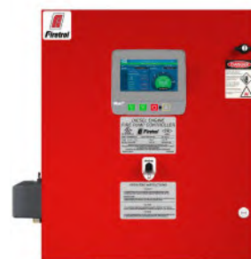
Diesel Engine Fire Pump Controller
